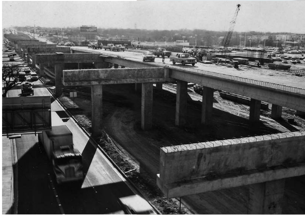
Construction of the upper deck of I-35 in Austin in 1972. The unique double deck construction of this stretch of roadway allowed lanes to be built in this tight stretch of Austin. (courtesy of TxDOT)
