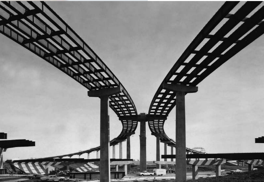
Construction of the I-35 and I-635 interchange in Dallas. The major cities in Texas built loops, such as I-635, around the central core of the city as a practical way of navigation and congestion relief. (courtesy of TxDOT)
