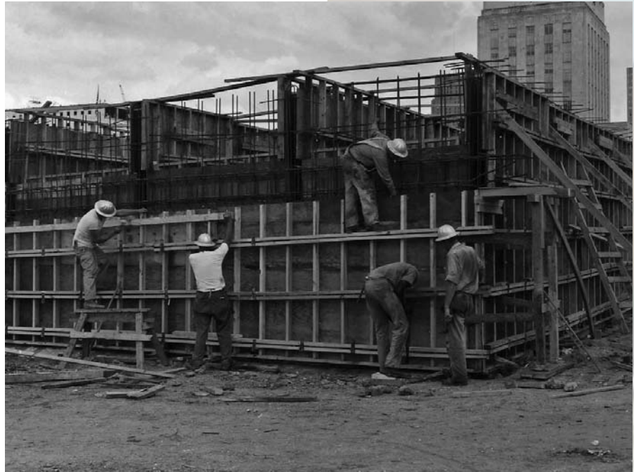
Workers build a frame during construction of I-45 in Houston in 1961. (courtesy of TxDOT)
