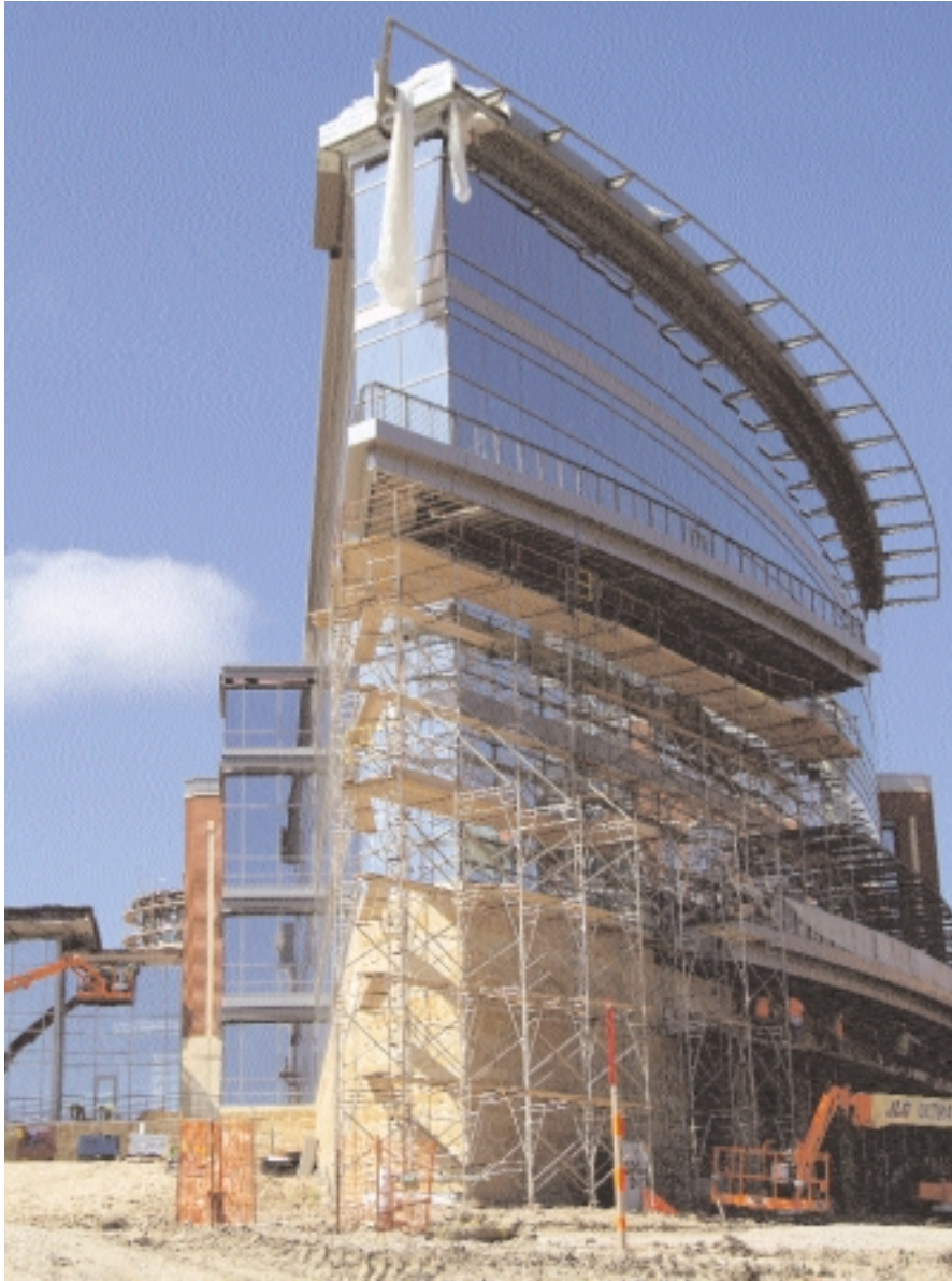
LEFT: The jackknife edge of the commons building features an employee dining room and, above, a conference room, both with a panoramic view of the Trinity River. (Photo © John W. Davis, ASMP Dallas Visual Design)
