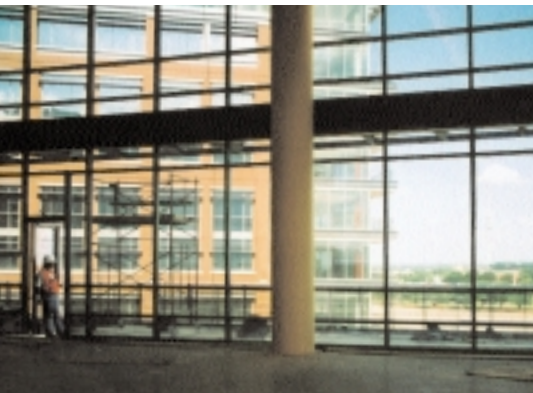
TOP: Two of the three office buildings will overlook green space on three sides and exhibit the traditional masonry design that complements other buildings in nearby downtown Fort Worth.
