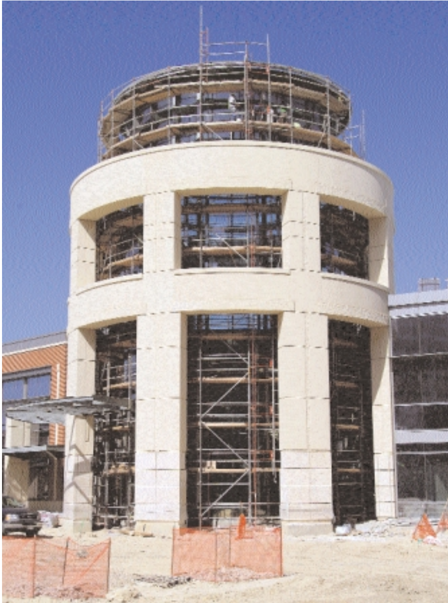
LEFT: With scaffolding still in place, a four-story rotunda of pre-cast stone and glass takes shape at the main entrance. (Photo © John W. Davis, ASMP Dallas Visual Design)
